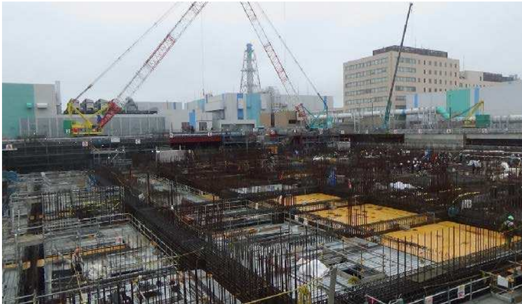
Figure 2: MOX Fuel Plant Construction June 2023 at JNFL 1 site (credit Japan Nuclear Fuel Limited).
