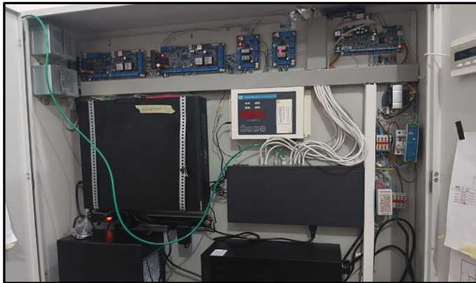
Figure 1: Cabinet Installation with ATS Controller including Extensions with NVR, LUDLUM
