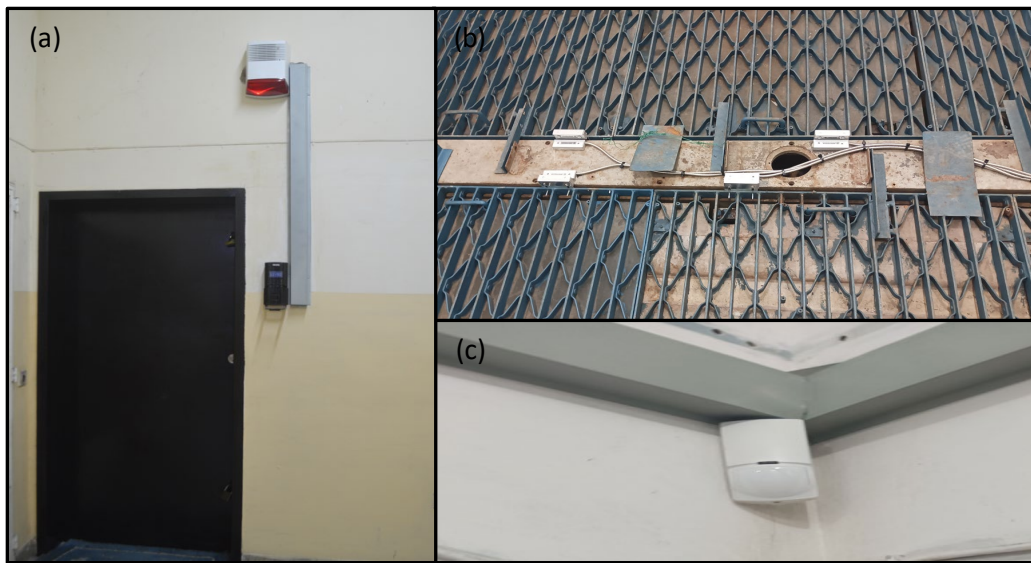
Figure 3: Deployment of secure magnetic metal doors with Cameras and palm reader (a), Motion Sensor and BMS installation (b and c)
