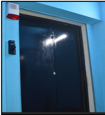
Figure 5: Deployment of secure magnetic metal doors with palm reader, camera inside the TRICO II hall
